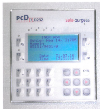
Zwei SAIA PCD3-Stationen regeln die komplette Anlage. The Entire system is regulated by two SAIA PCD3 stations.
